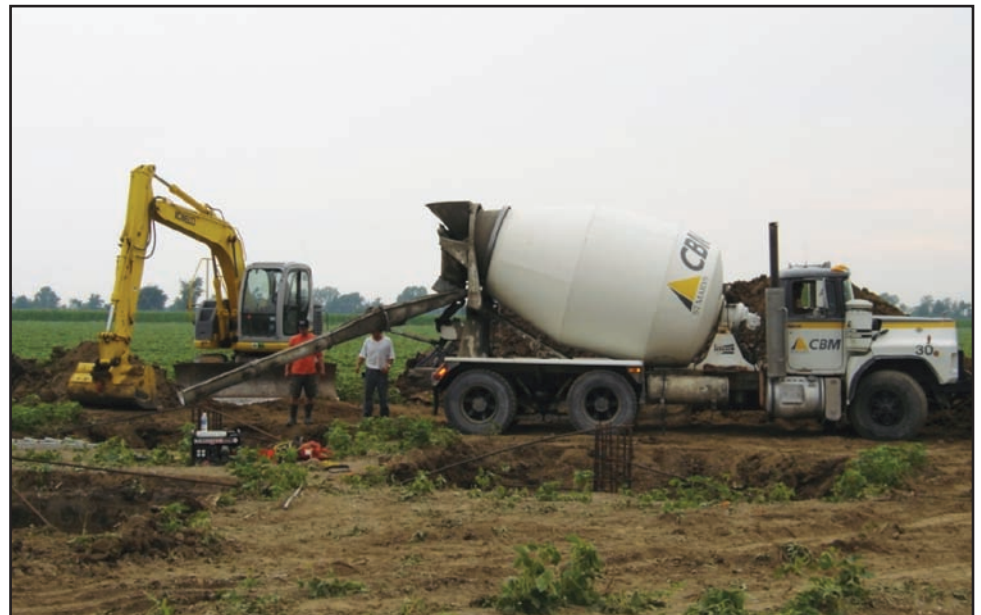
July, 2007 - Cement is poured during the construction of the permanent wind measurement mast base.
